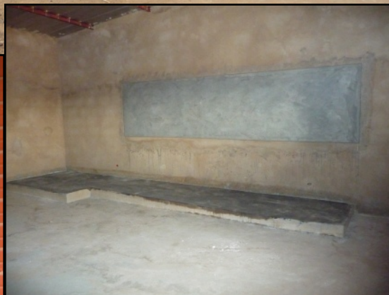
Inside the classroom; blackboard, & elevated place for the teacher and desk. The blackboard will get a coat of black paint.
